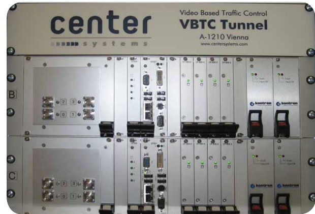
Fig. 4: How VBTC Tunnel's VESA units are constructed, from left to right: PCI-based frame grabber cards, a RAID controller, a Kontron CP307 CPU board, four hard-drive slots, and two power supply units
